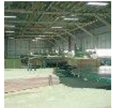
Thirteen Raimann patchers are installed in two lines. Rotary sorting table at right.
